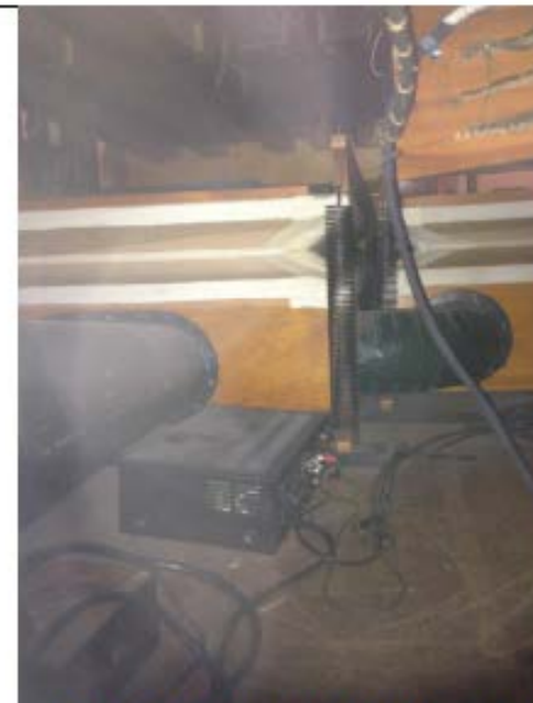
Figure 6: Two air reservoirs on the floor. The small box is a DC power supply (there is another in the basement by the blower).
